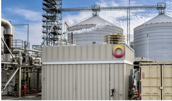
Rondo heat battery at Calgren site
